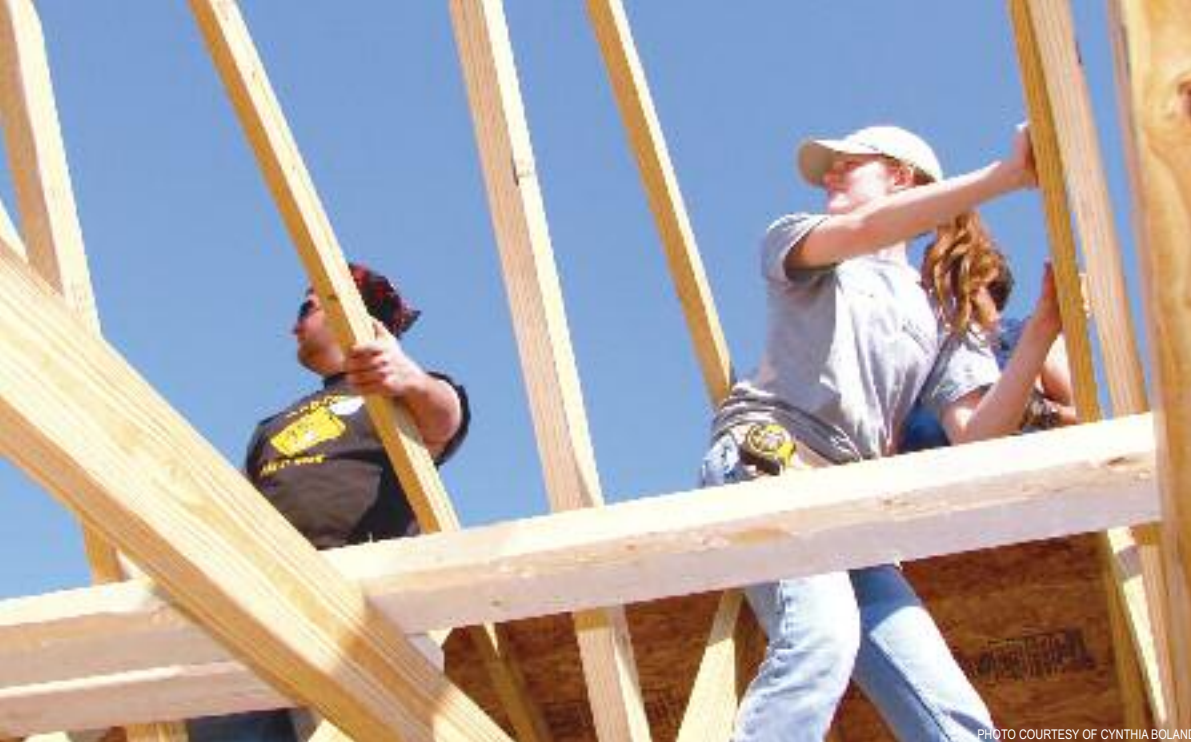
Left: Seton Hill students Scott Karan, '07 and Andrea Denniston, '07 help build the roof of a new house in Birmingham, Alabama during Campus Ministry's 2007 Spring Break Habitat for Humanity trip.
